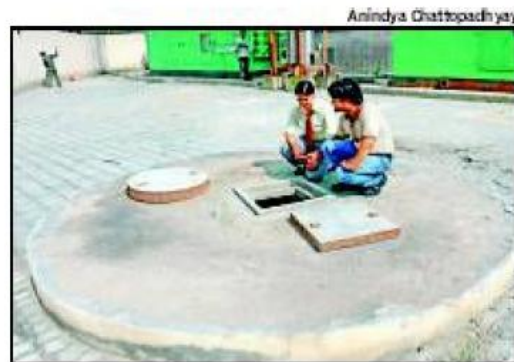
Few stations and depots have rainwater harvesting
