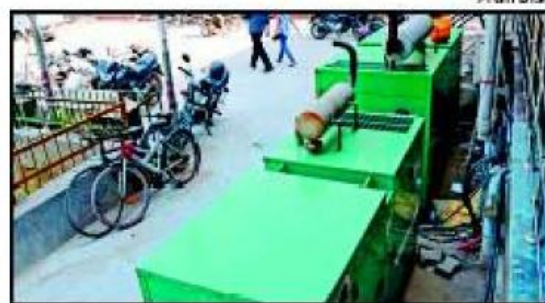
Heavy duty generator sets are posing a health hazard
